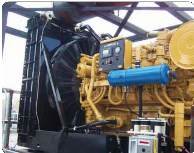
Pump Emergency Shutdown
