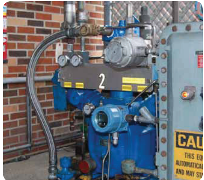
Gas Compressor Protection
